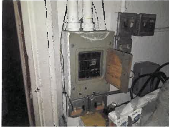
Figure 3. Federal Pacific Panel in Projector room.
