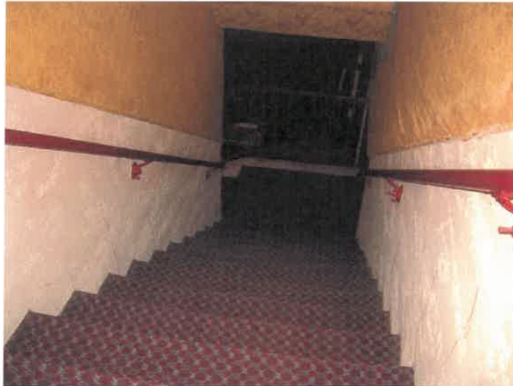
Figure 3. The existing stairs do not meet current code requirements for egress and accessibility
