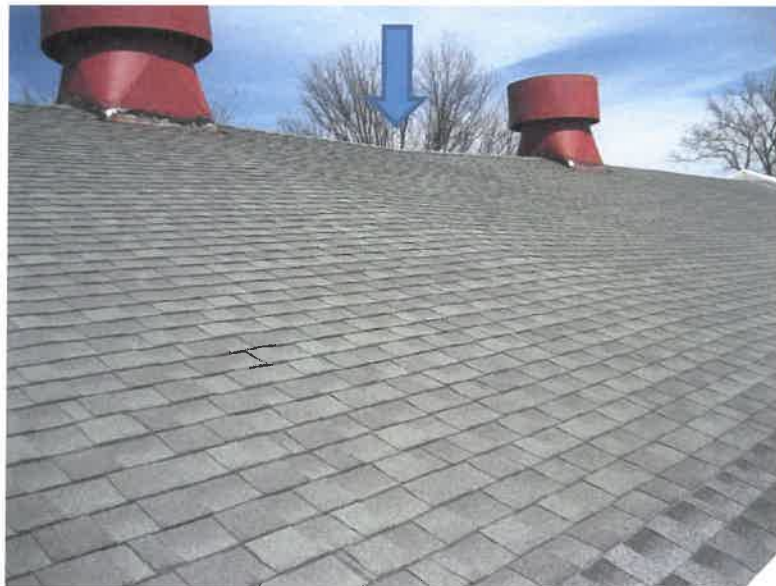
Figure 13. Depressions in Roof at Truss Damage
