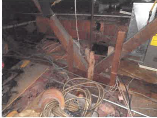
Figure 11. Typical disorganized, unsupported/unsecured wiring in attic space.
