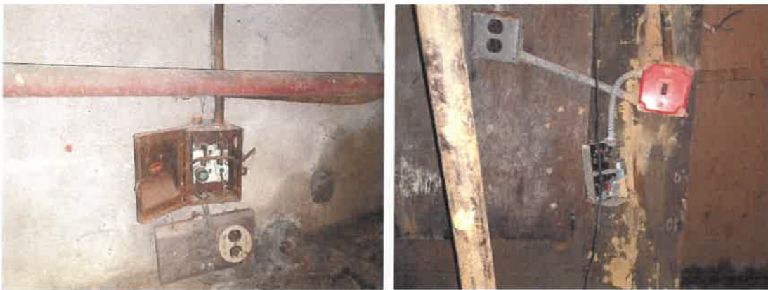
Figure 12. Typical corroded/abandoned devices in old boiler room.
