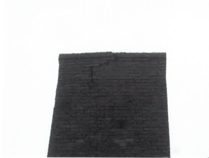
Figure 7. Significant Crack and Displacement of Masonry Chimney at Southeast Corner
