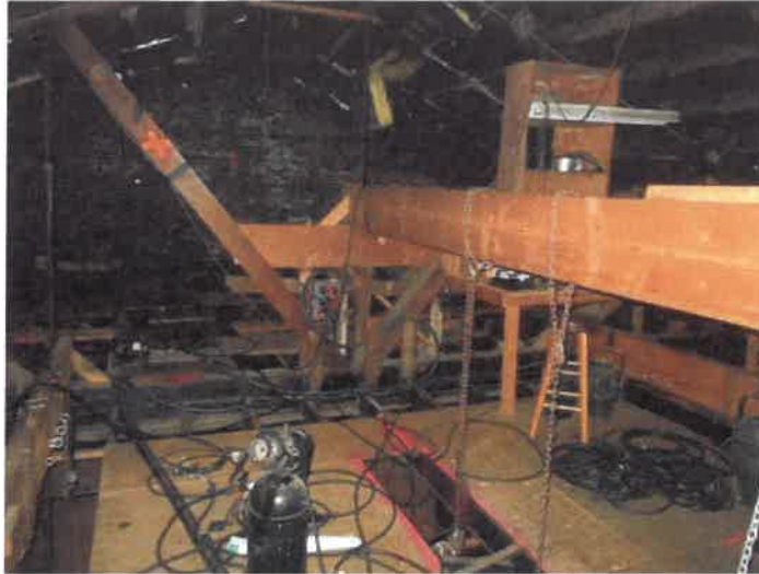
Figure 5. Stage Lights and Prop Hoisting Equipment on Inadequately Sized Attic Joints (Note Lack of Guardrails and Openings in Floor Creating Workplace Hazards)
