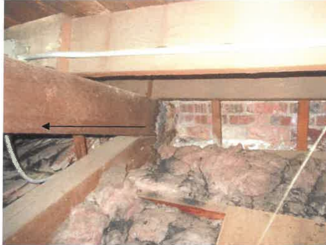
Figure 2. Timber Truss with Moisture Damage at Bearing Location (Exterior Brick Wall in Background)
