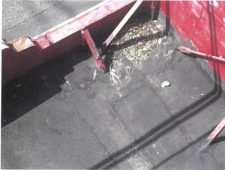
Figure 16. Debris Accumulation and Use of Roof Cement for Flashing
