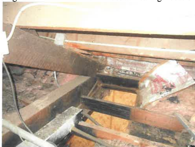
Figure 4. Severely Cracked and Displaced Roof Truss at Exterior Wall Support
