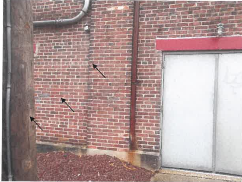
Figure 5. Cracked Brick Masonry (North Elevation)
