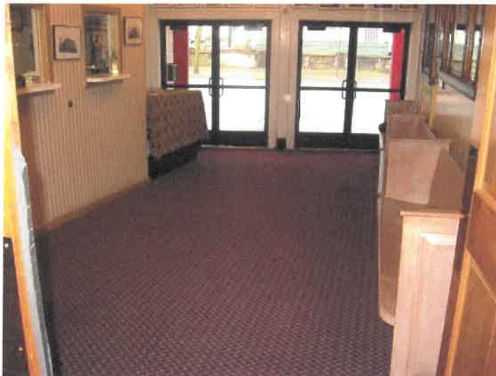
Figure 1. The entry lobby floor is continuously sloped. The floor would need to be level at the entry doors and in front of the ticket window. Elevation changes do not appear to be able to be met with level surfaces.
