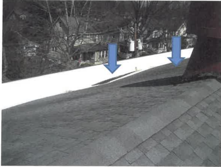
Figure 14. Depressions in Roof at Truss Damage
