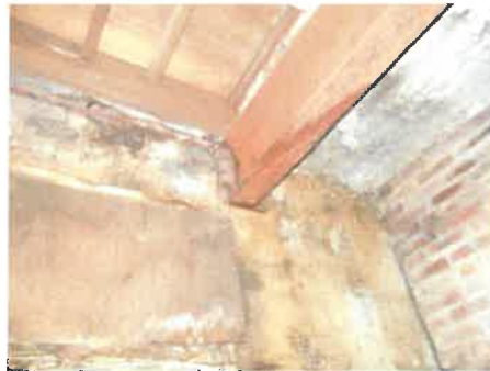
Figure 1. Localized Corrosion of Steel Framing at Rear/East Foundation Wall
