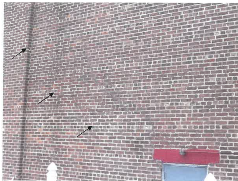
Figure 6. Cracked Brick Masonry (South Elevation)
