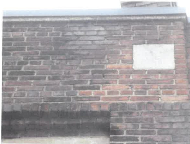
Figure 4. Deteriorated/Open Joints at Parapet Wall (Front/West Elevation)
