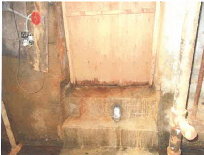
Figure 10. Water Infiltration at Cellar Level Through Abandoned Exit
