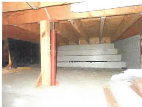
Figure 2. Wood Stage Framing (Joists Over-spanned for Required Loads, Improper Girder Dimensions, Improper Support Post Anchorage, Note Temporary Steel Shore Post in Place)
