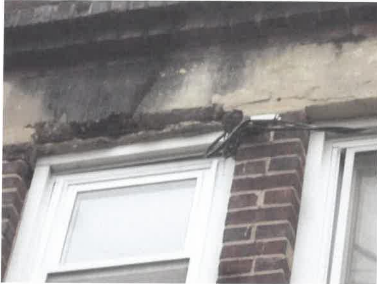
Figure 3. Spalled Concrete Lintel at Front/West Elevation Typ. 3 Locations (Balcony Level)
