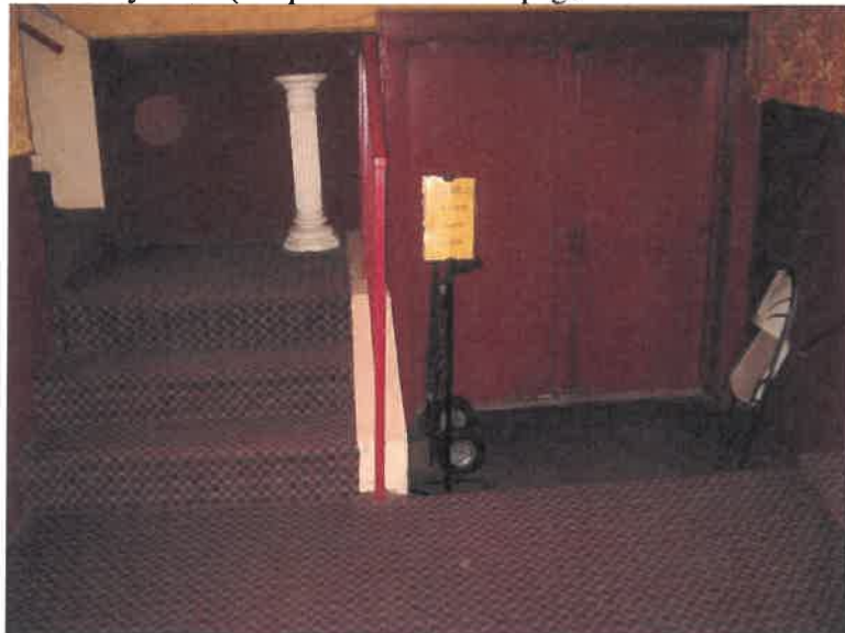
Figure 4. This emergency exit does not meet current code requirements for egress.
