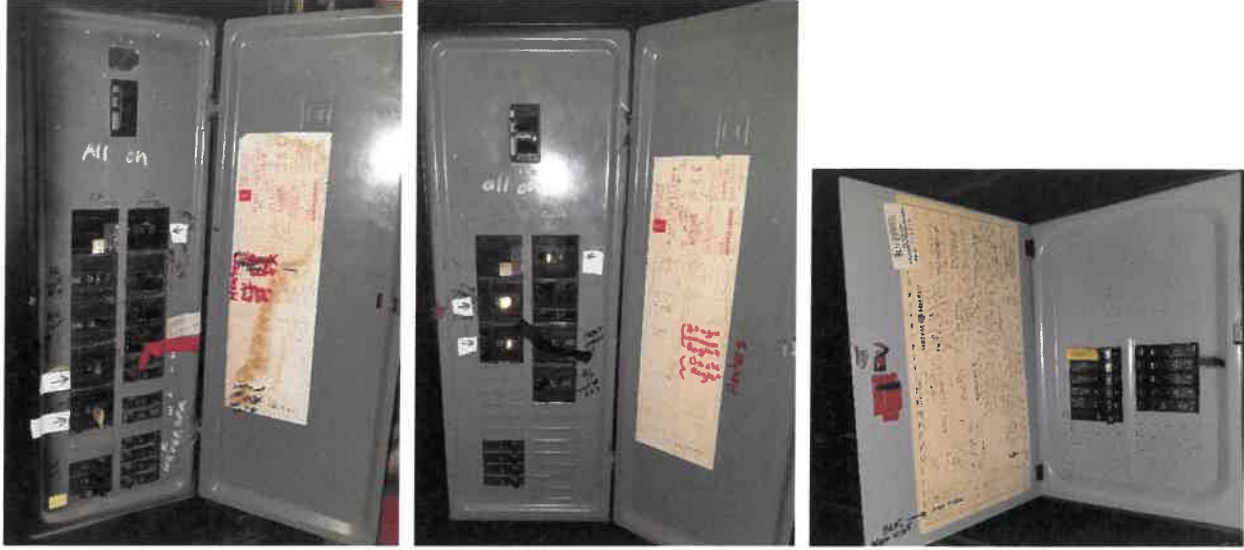
Figure 7, 8, and 9. Panels at electrical service entrance in stage area.
