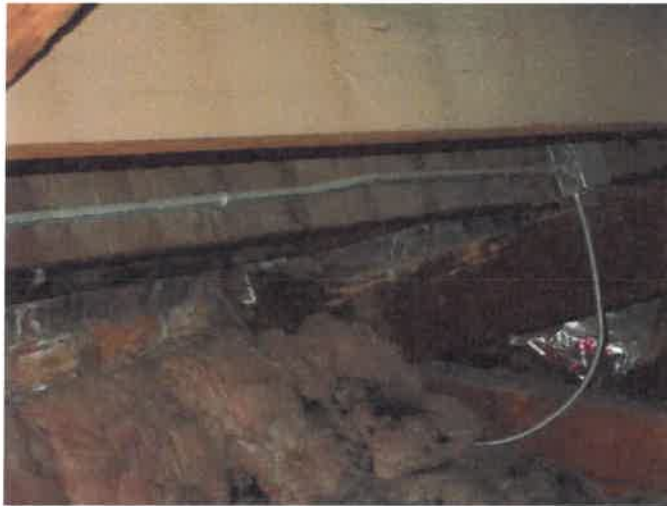
Figure 3. Cracked Timber Truss at Bearing Location
