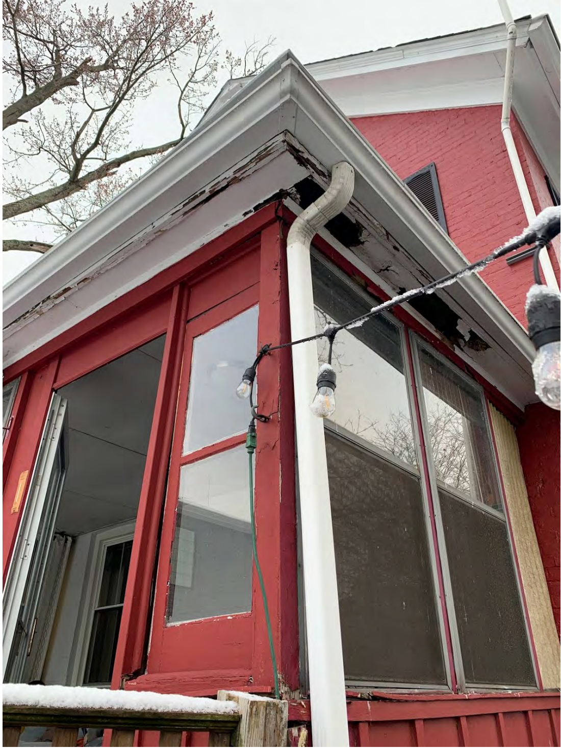
Evidence of porch deterioration
