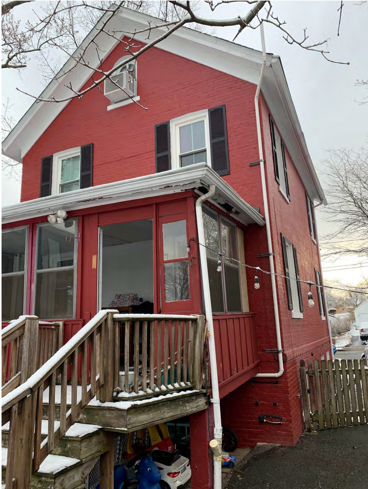
Rear corner of house where proposed work would cross side set back.
